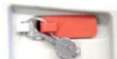
Locked with Wire Seal
